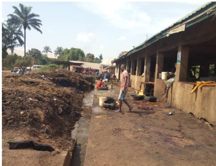
Plate I: Side view of Ikpa slaughterhouse, Nsukka. Both solid and effluent were accumulated beside the kill floor. Butchers usually slaughter on the ground floor which are already in a dilapidated condition. No adequate water supply as water is source with containers
