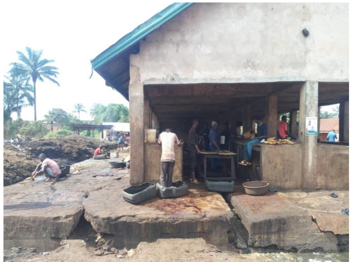
Plate II: Front view of Ikpa slaughterhouse, Nsukka showing the dilapidated condition of the kill floor and the effluent disposal channel
